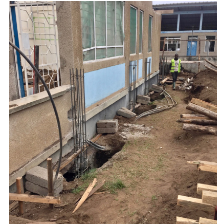
Selian Hospital Lab construction is underway. This is one piece of helping SLH achieve a higher level of accreditation.
